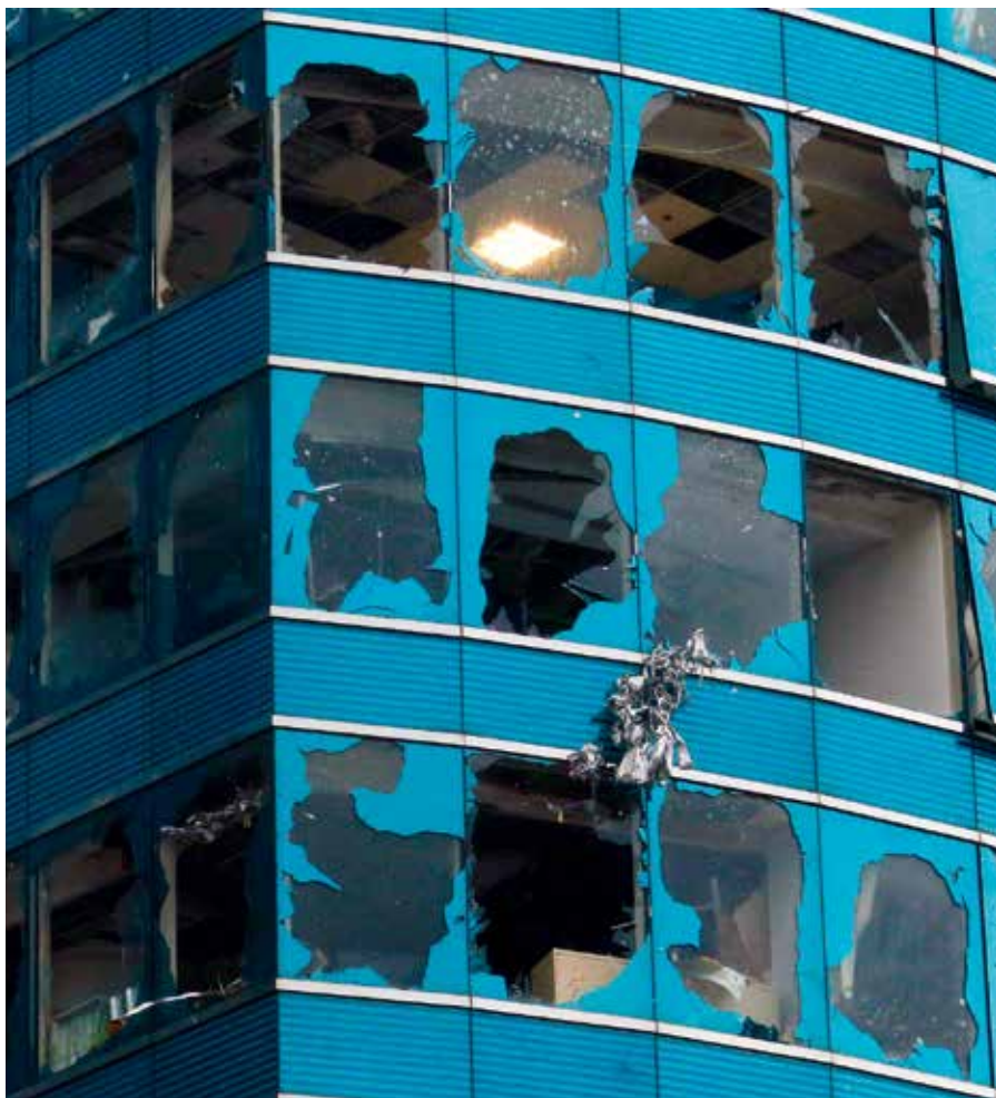
September 16, 2018: Damaged windows of a One Harbourfront office tower following Typhoon Mangkhut in Hong Kong. VCG
